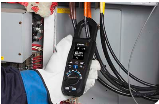
Verify amperage measurements
